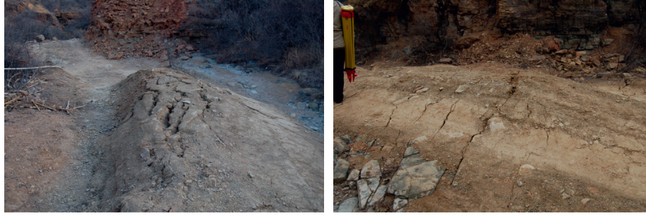
FIGURE 13: Point 2: fractures and uplift at the ravine.
