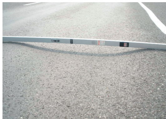
FIGURE 7: Result of the rutting survey at sample 5.
