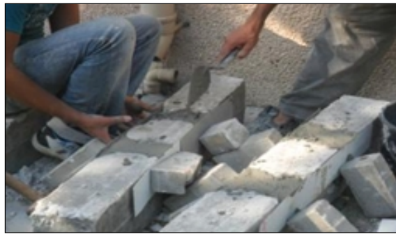
Fig. 4. Cracked beams after application of the repair materials
