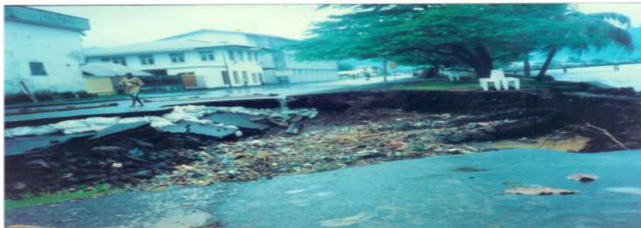
Figure 2. The main road at 'Down Beach' eroded by oceanic waves in June 2001
