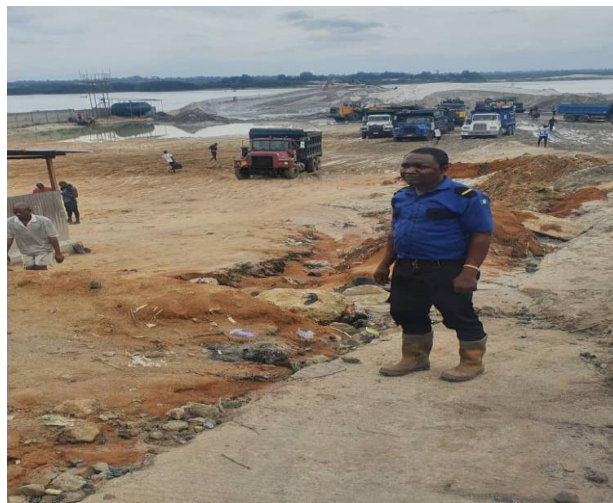
Plate 1. Heavy Erosion at Abuloma mining site. Source: Researcher's field work (2021)
