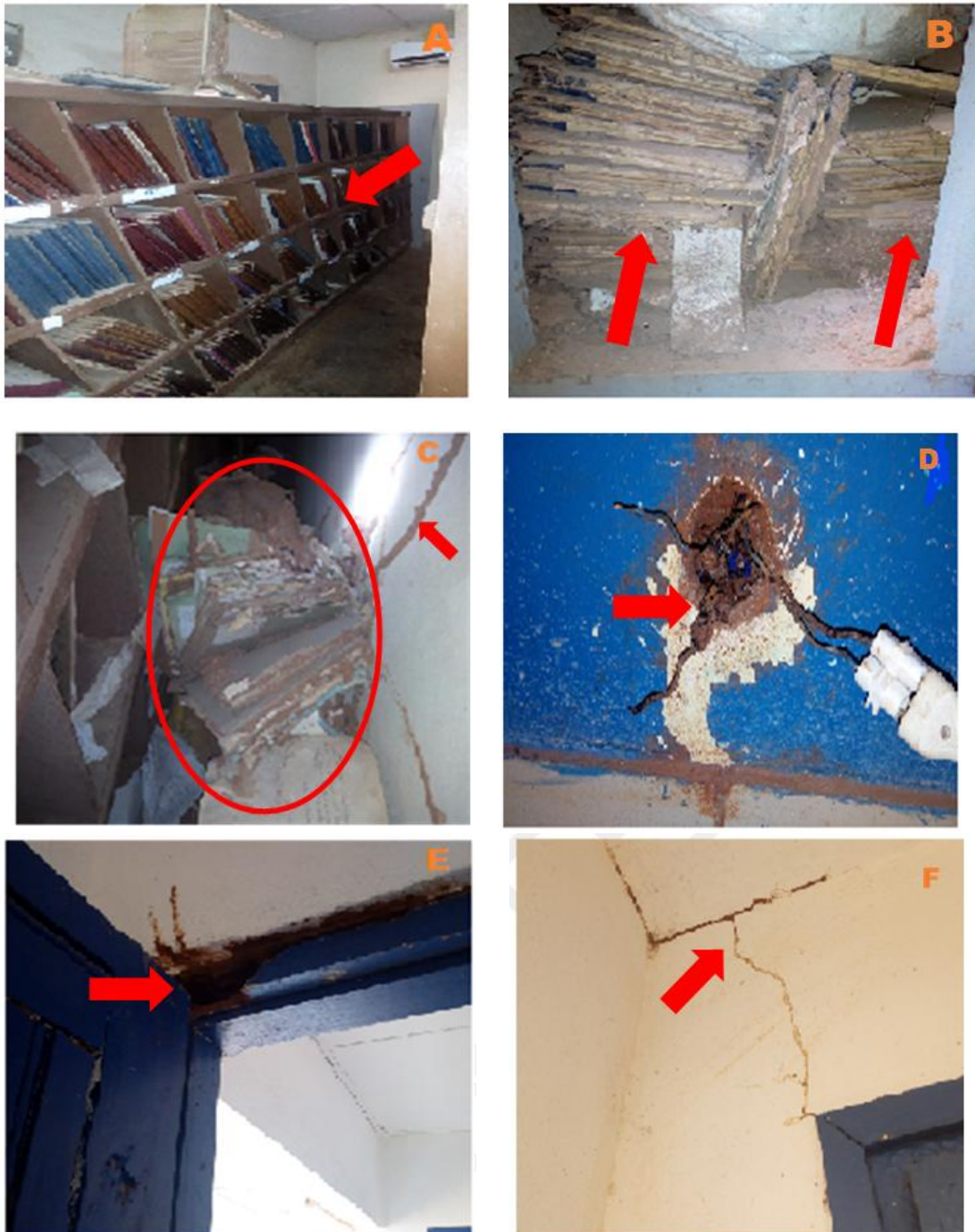
Fig. 3. Termite damage at investigation sites
